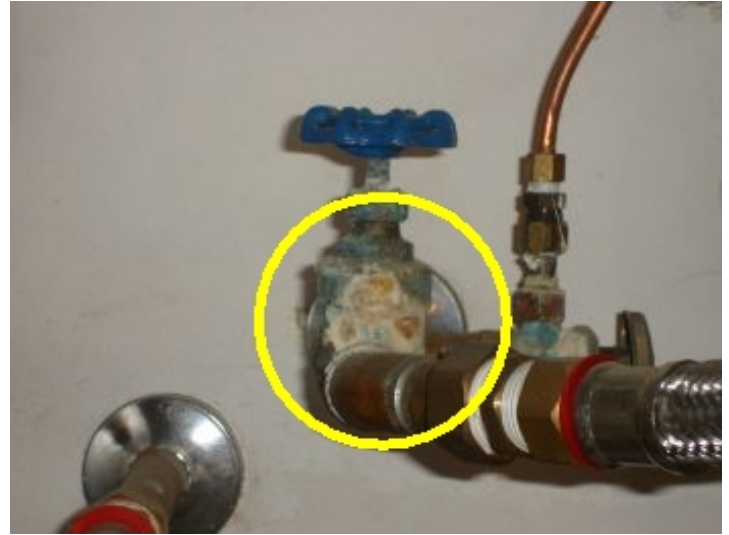
Calcified remains of previous leak
