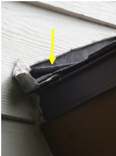
Undersized flashing, exposed sheathing
