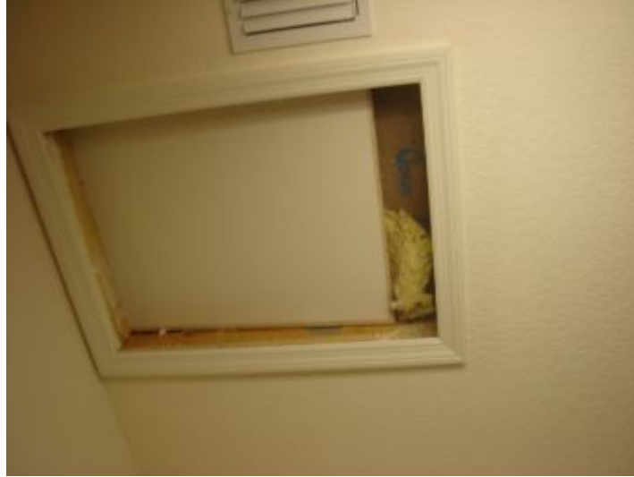
Blocked access to attic
