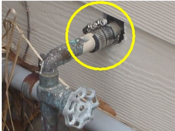
Unprofessional repair. Water Main shutoff
