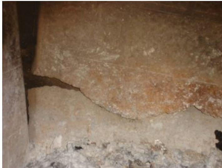
Damaged rear refractor
