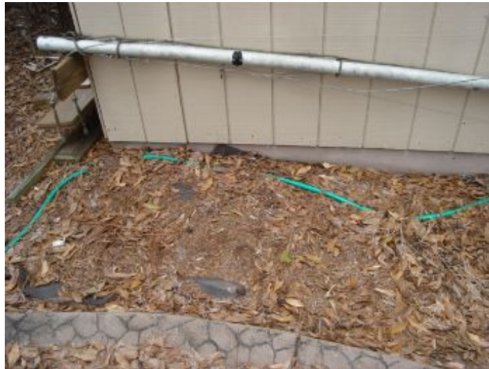
Grade is too close to siding, may cause moisture to wick into siding.
