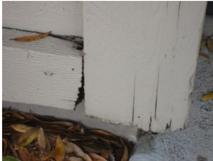
Dry rot in exterior trim
