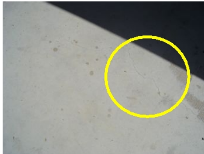
Minor settlement cracks in rear Lanai
