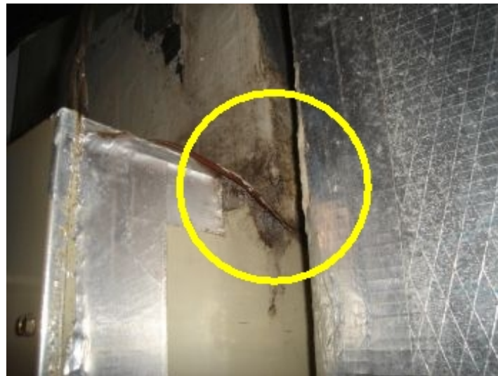
Organic type material on exterior of air handler
