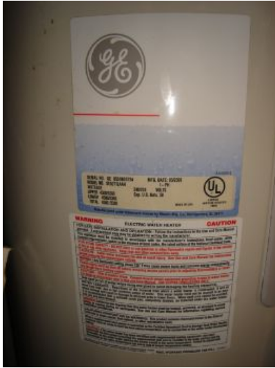
Water heater data plate
