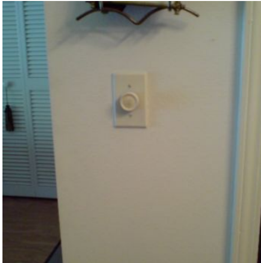
Dimmer switch in living area
