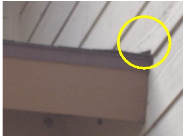
Missing kick out flashing on Northwest side of roof
