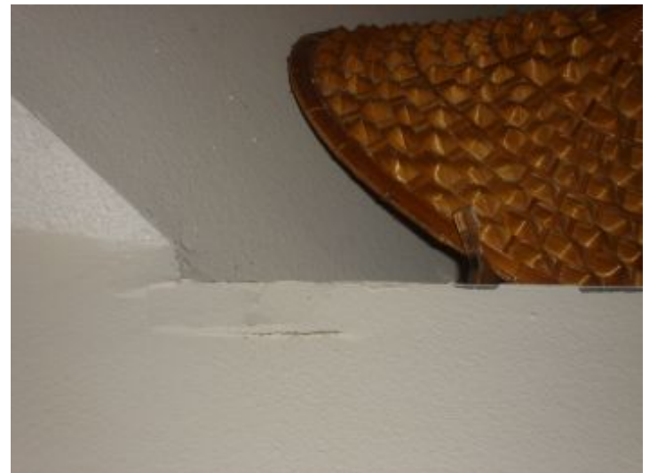
Detached/lifting tape seams
